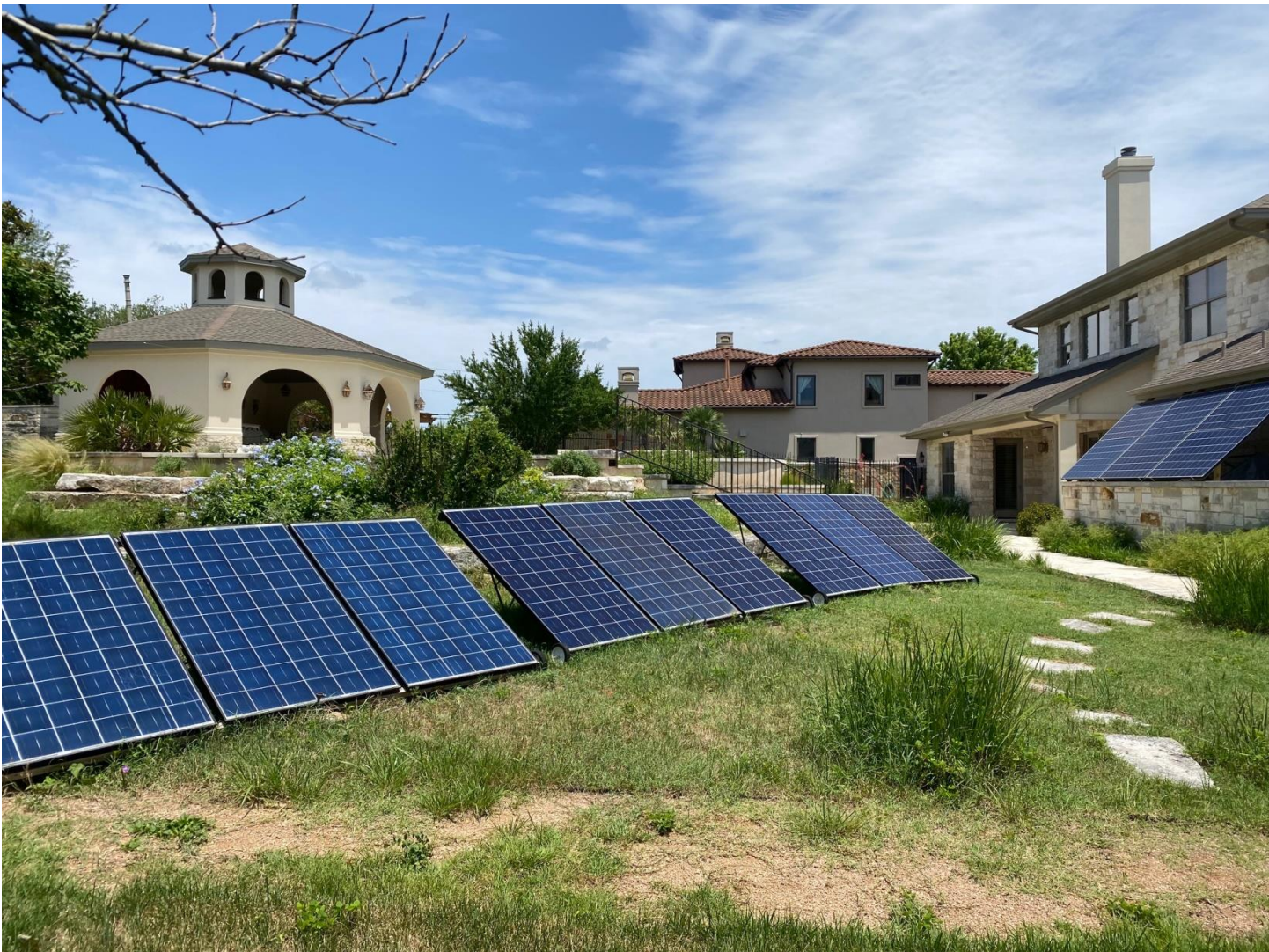
The ground mounted panels can be manually rotated to track the sun.
